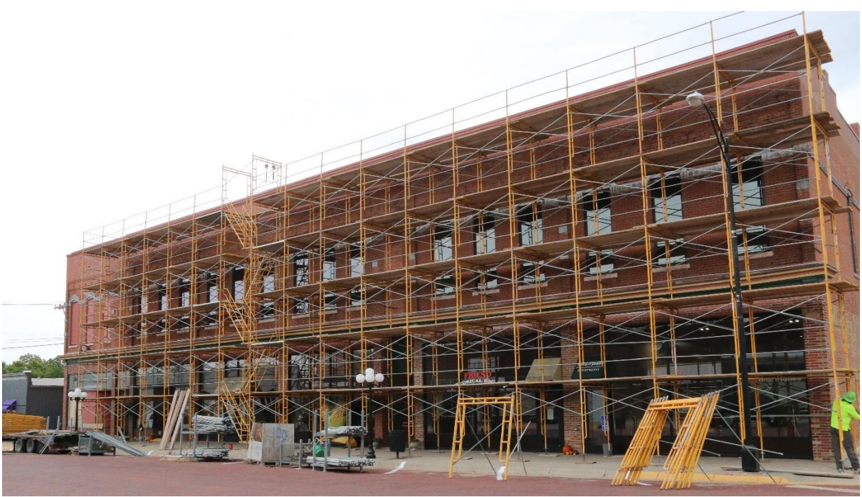
The first phase in the Shovel Ready Grant, scaffolding on the north and west sides. This picture was taken on October 4, 2022. The grant funded new brick, cap flashing, helix ties, tuck pointing, north foundation repair, steel beam under the Welcome Center, etc.
